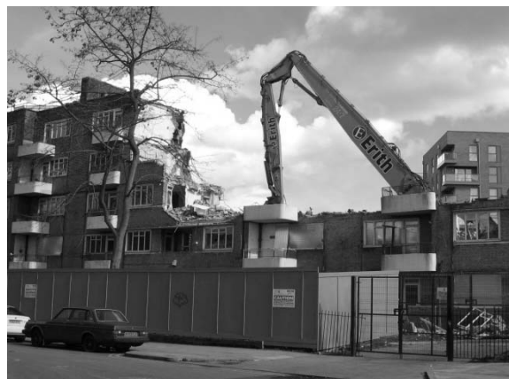
Watch 'em come down – demolition of the last 1938 blocks on the Guinness Trust Estate in Loughborough Park (Bx-M16-06.jpg).
