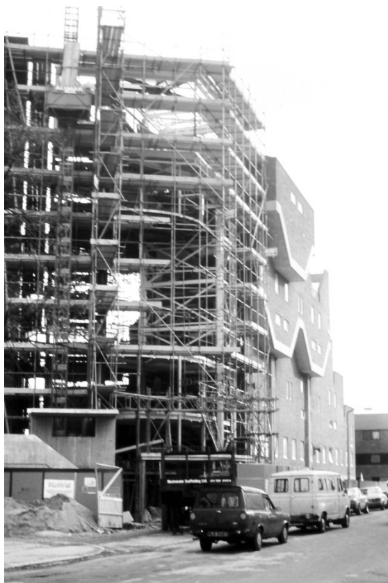
The Southwyck House "barrier block" being fitted with new lifts and entrances in 1991-92. (BS-EBx-92-03.jpg)
