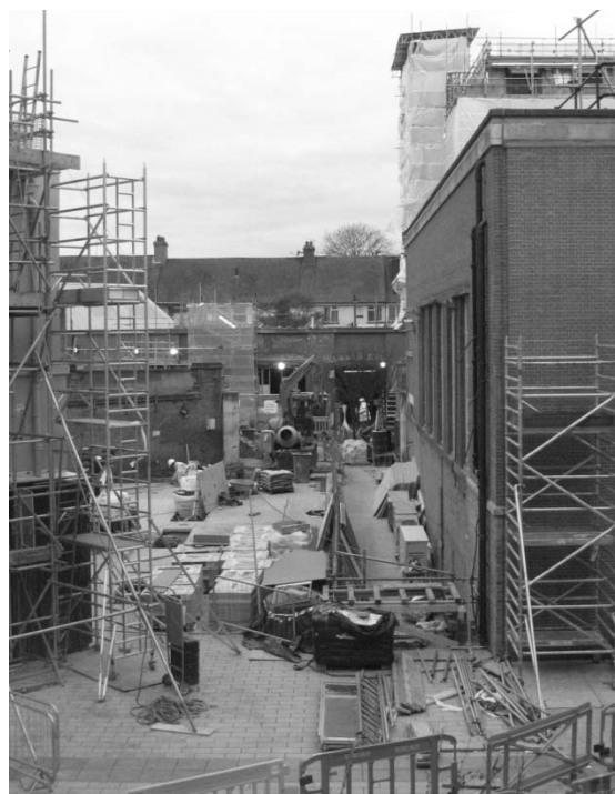
Rear courtyard under construction, to provide level access from Buckner Road; Also note the side wall of the Assembly Hall on the right, and Porden Road houses in the background. (BTC-TH17-06.jpg)
