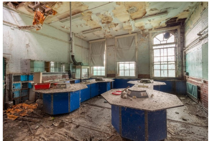
A decaying classroom. As bad as it looks, it does not necessarily imply there is structural damage.
